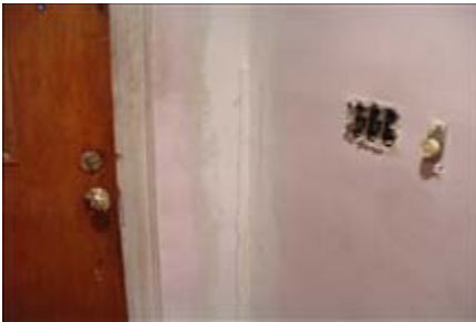
Note open access panel
