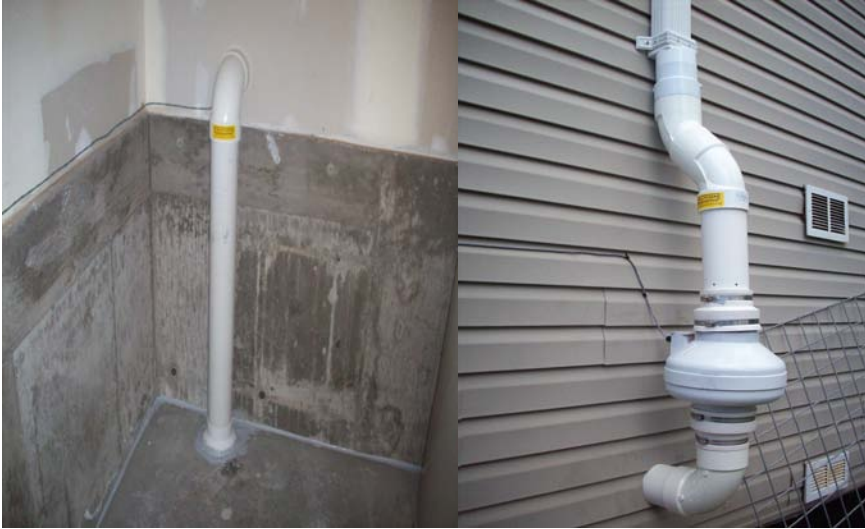
(Piping connected to hole in slab; fan attached to piping on exterior)
