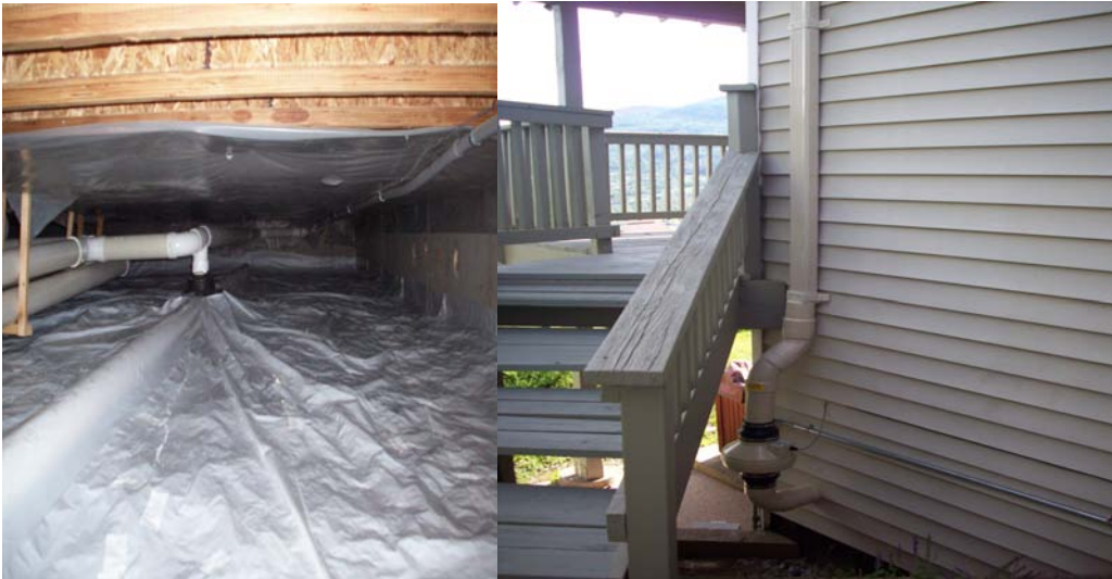
(Radon barrier covering soil & perforated piping in crawl space; fan attached on exterior)
