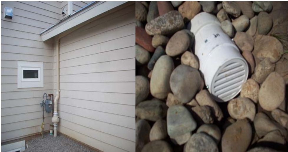
(Fan is connected to perimeter drain pipe; one-way valve installed on day light drain)
